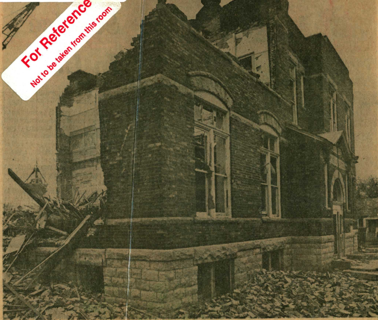
Time, safety hazards and the wrecker are leveling the Indiana School.
